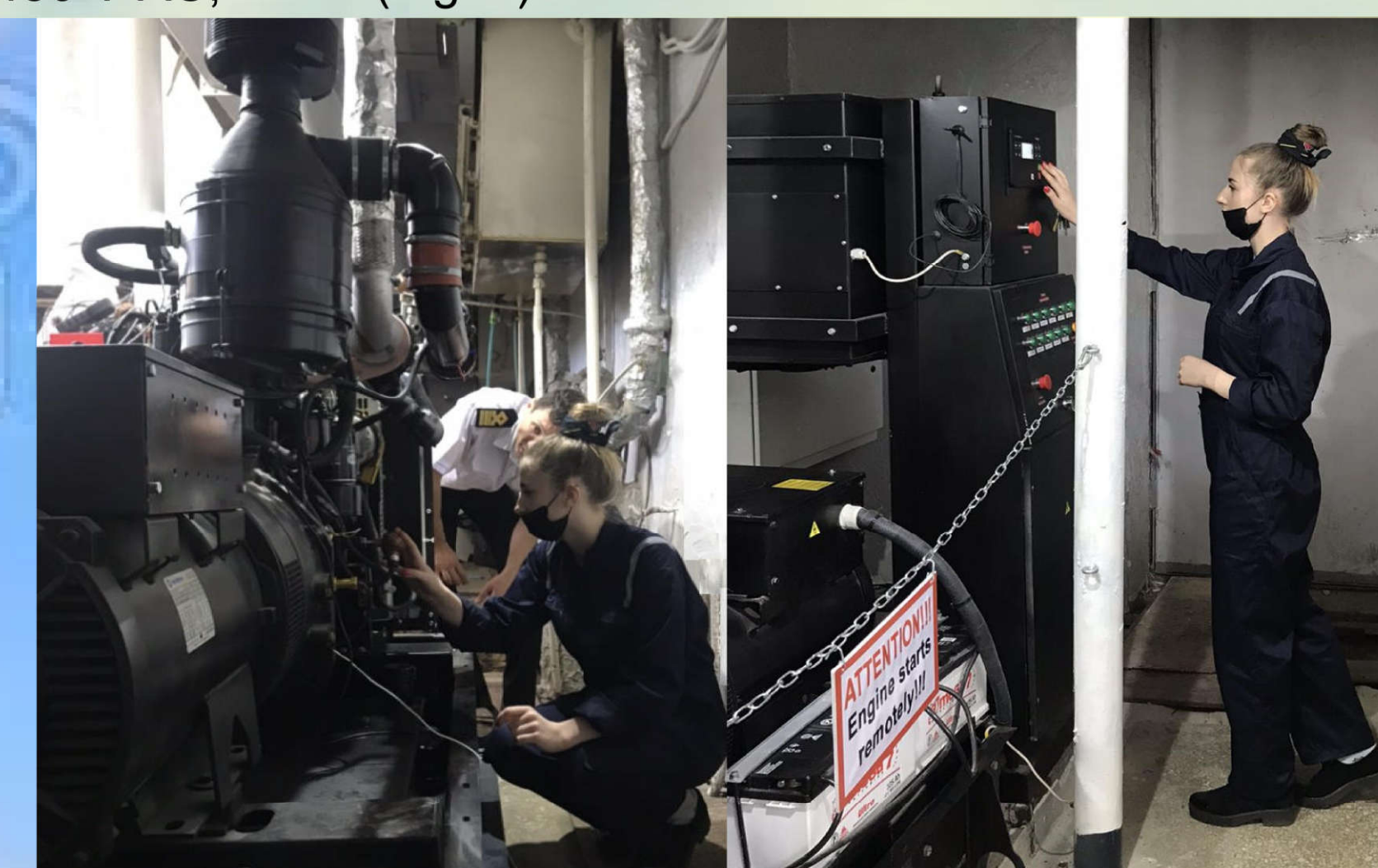
Figure 3. Participant in the real conditions preparing to start and start emergency diesel generator in the academic engine room laboratory
